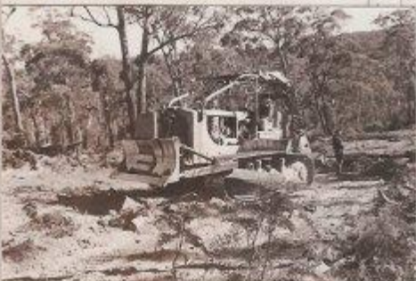
Greg, our dozer driver, led by George, finishes clearing the dirt circuit.
